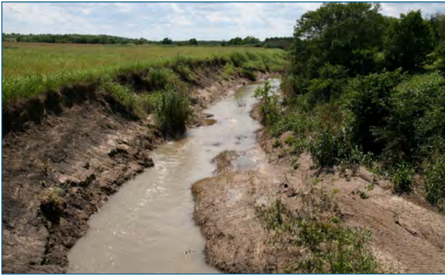
This stream is experiencing excessive erosion.
